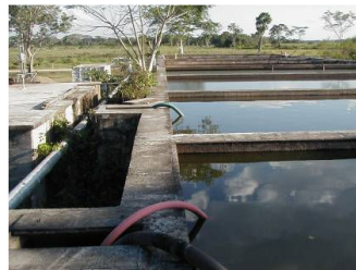
Bypass hose in slow sand filter basin
