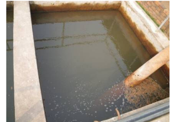
Bypass hose also in rapid filter basin
