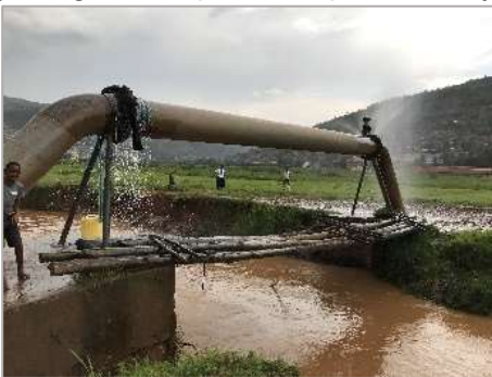
Leakage from the largest transmission pipe
