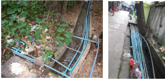
Figure 2 Several service pipes in parallel on the ground
