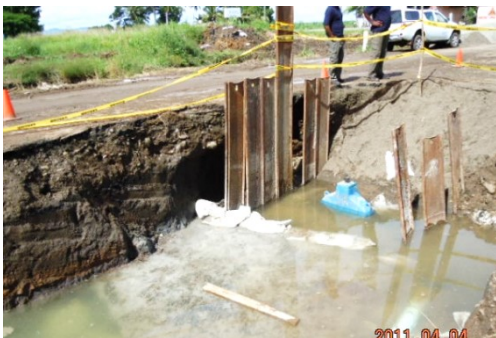
Photo 3: Underground water flowing into pipe
