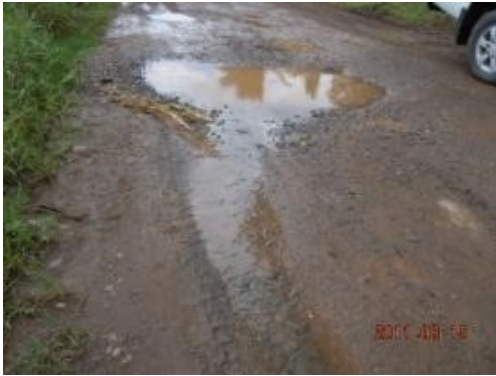
Photo 1: Leakage on the ground
