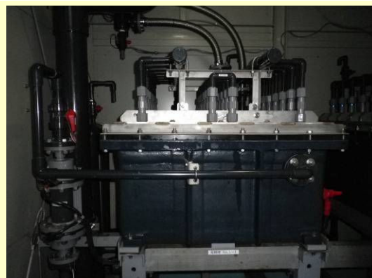
Electrolysis tank of NaClO generator
