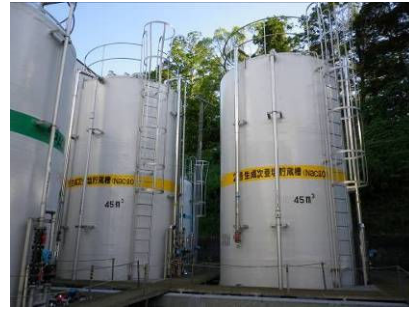
NaClO storage tanks
